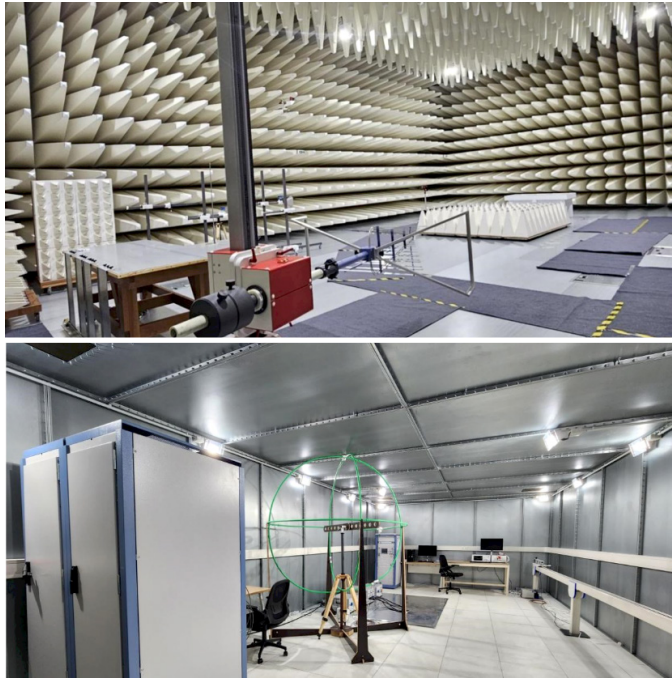
Gambar 3.18 EMC Chamber 10m dan Shielded room EMC Test System (EMI) - Conducted Emission
